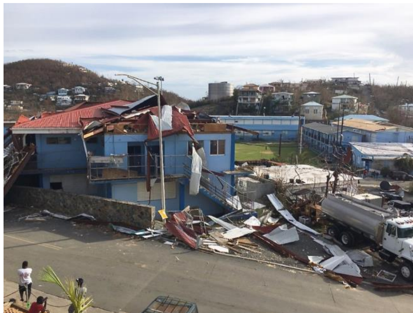
Figure 4.33: Sprauve School Annex after Irma finished tearing it apart in St John. (Amy Roberts, St. Thomas Source, September 9, 2017)
