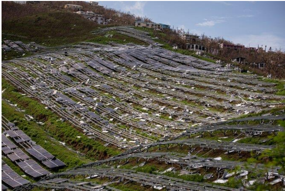
Figure 4.32: Solar panels that provided a small percentage of power for St. Thomas were destroyed (Hilary Swift for The New York Times)
