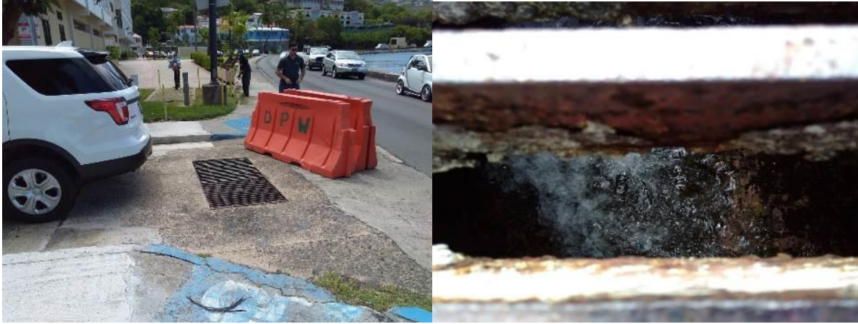
Figure 4.31: During high tide events, seawater can impede proper drainage of urban centers. Stormwater drain in Charlotte Amalie (left); closeup of wave travelling upstream in drain at low tide (right).
