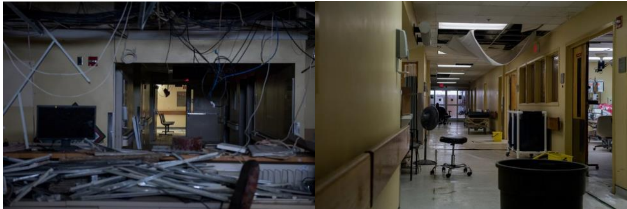
Figure 4.11: Hospital Severely Damaged from Hurricane Irma (Hilary Swift for the New York Times)
