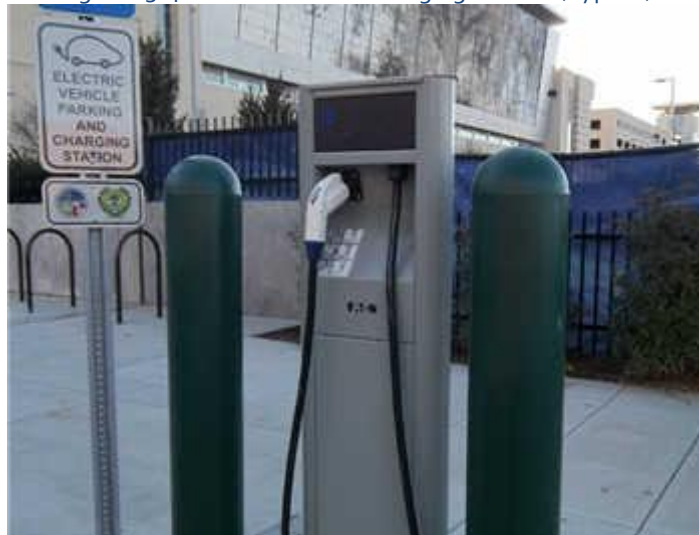
Figure 13-4: Electric Vehicle Charging Station (Typical)
