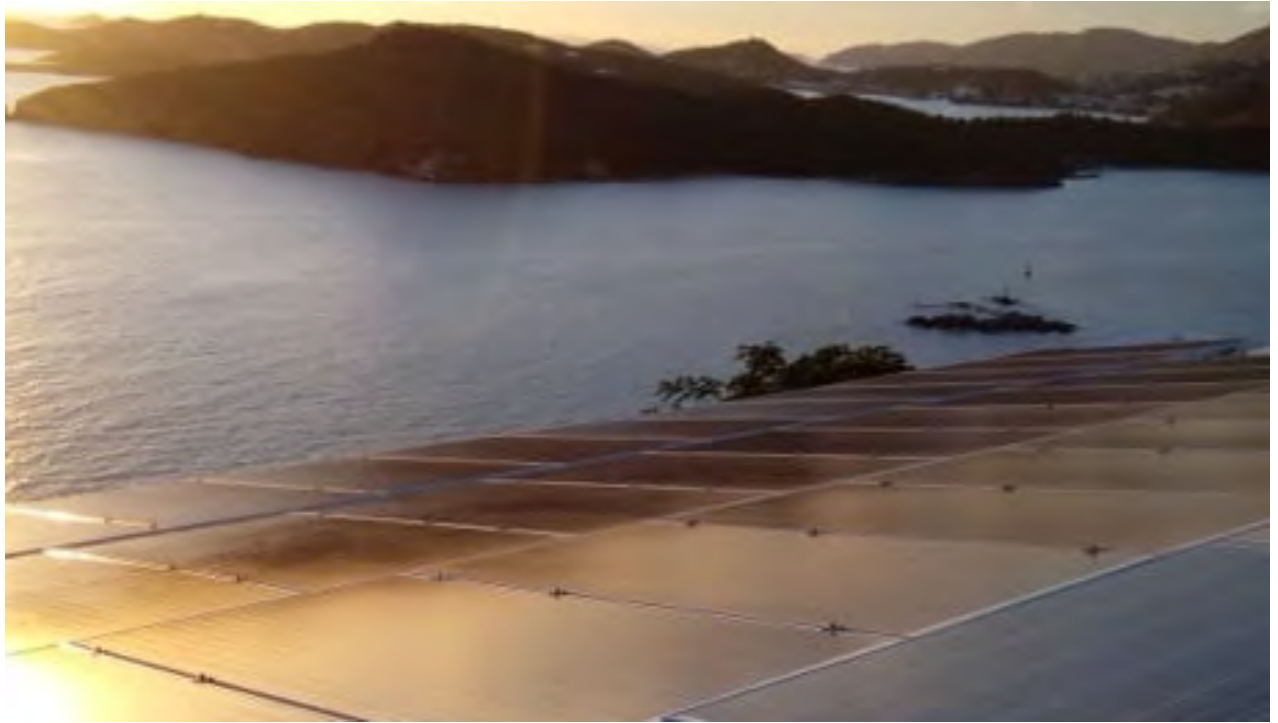
Solar installation in the U.S. Virgin Islands
